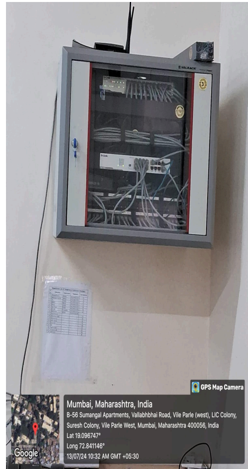
(Networking Distribution Switch Room No. 3.8)
