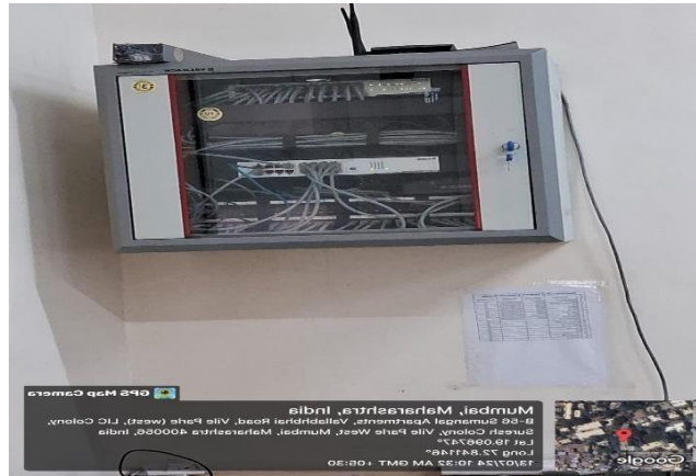
3.8 Networking Distribution switch
